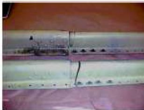
Substructure – Longeron Crack
